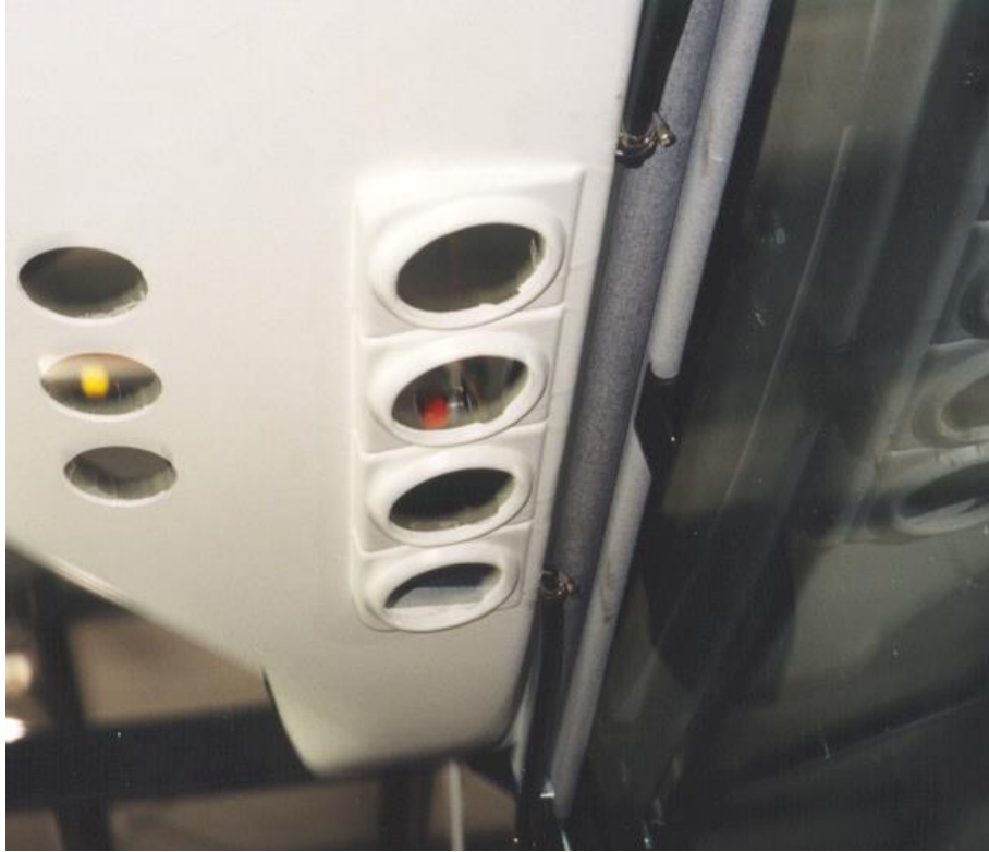
Drain tubes running along underside of headliner.
